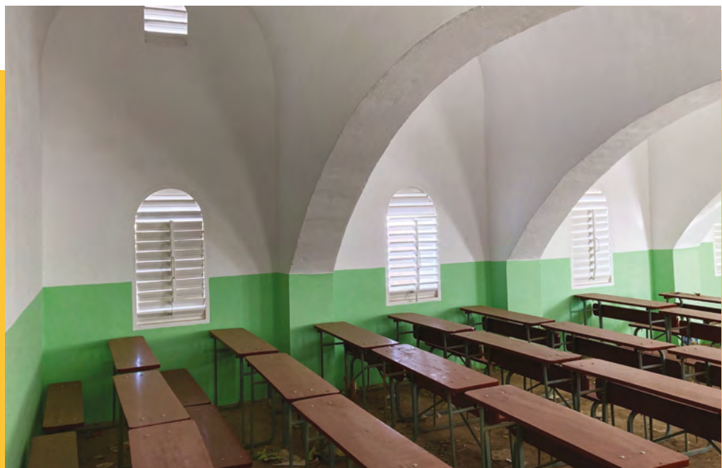
Open space between the vaults thanks to solid concrete block arches for a classroom with a length of 9m50 and a width of 6m50.
